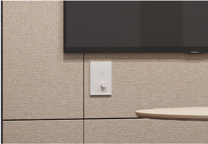
Manual control of ventilation and lighting
