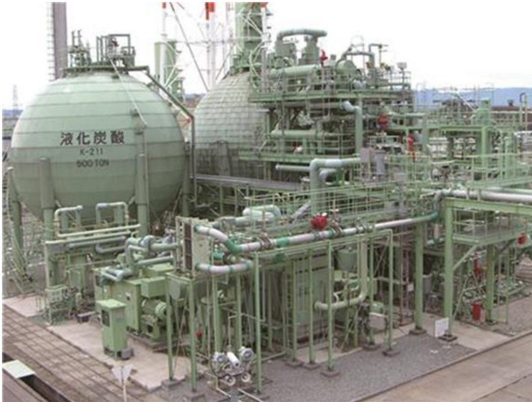
Figure 22: Carbon Dioxide Liquefaction plant at Senboku Terminal I. Photo courtesy of Osaka Gas
