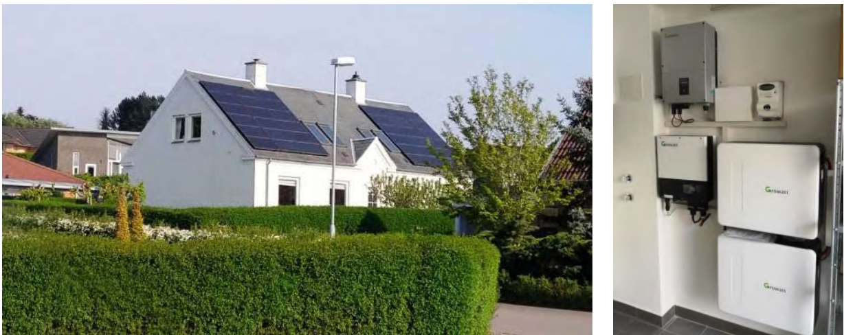
Denmark, Middelfart 3.6kW, Growatt SPA 3000TL
