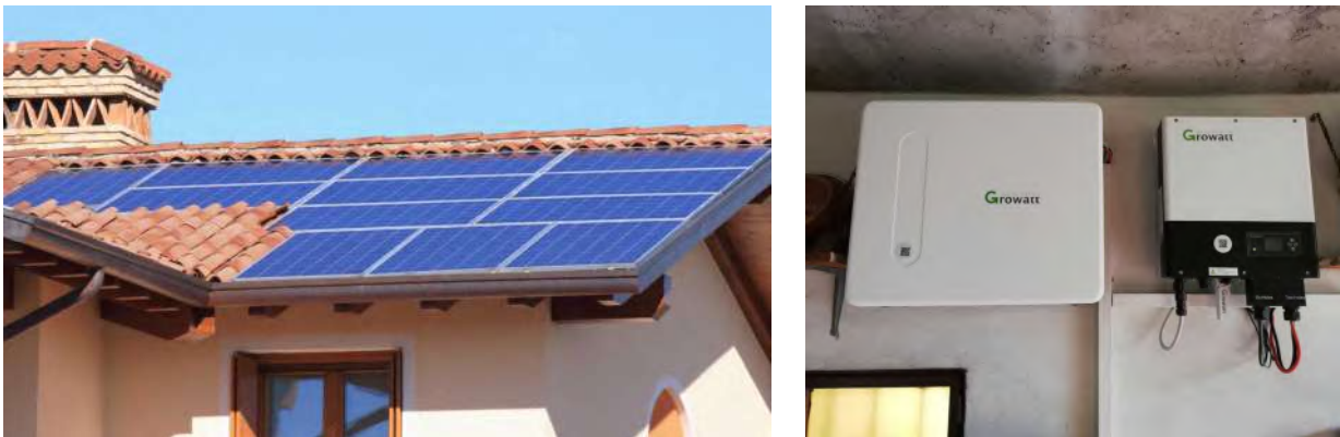
Italy, Milan 3kW, Growatt SPA3000TL BL
