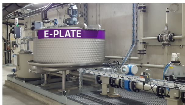
Heat Exchanger in a Wastewater Treatment Plant Inflow
