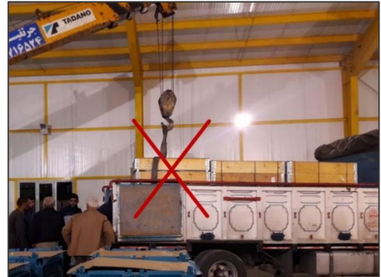
Figure 7: Wrong unloading of pallet box
