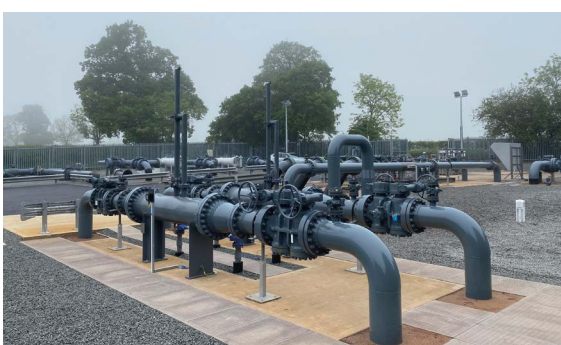
Example of equipment used at HAGIs
