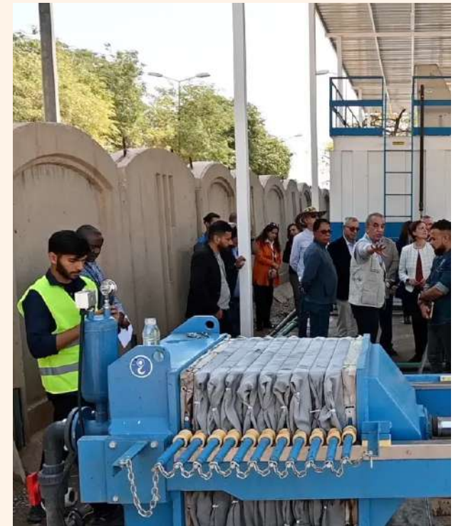
UNICEF and the United Nations Assistance Mission for Iraq (UNAMI) collaborated to install an MBBR wastewater treatment system at the UNAMI office building. MBBR systems installed across Iraq help reduce water shortages worsened by climate change. ©UNICEF Iraq
