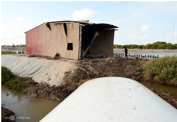
100-ton wind turbine blades fall to pieces in Vietnam - VnExpress International 18-12-2025
