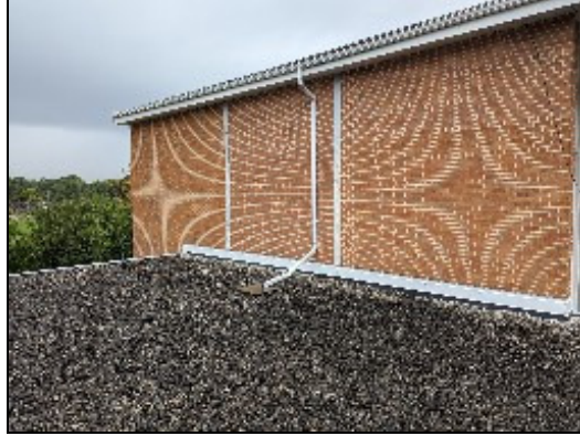
10. Downspout BLDG-3 drains onto Flat roof of BLDG-4
