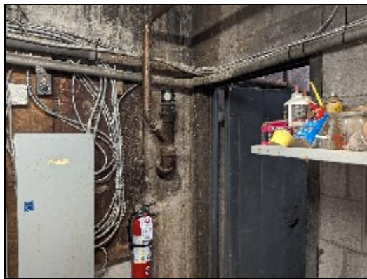
12. BLDG-3, sump pump-1 outlet pipe
