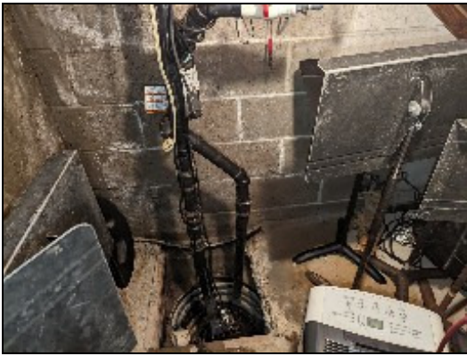
5. BLDG 5, Sump Pump -2 connects to combined sewer
