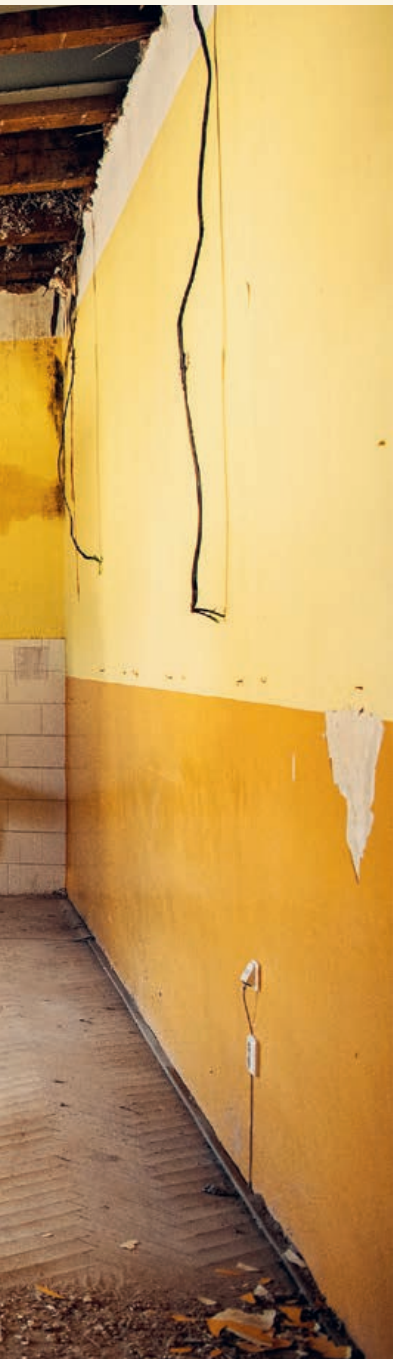
Tornado-damaged primary school in Moravská Nová Ves
