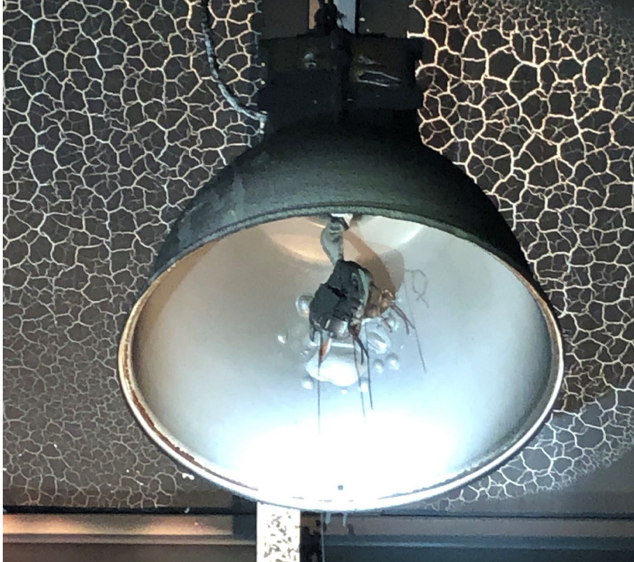
All lighting fixtures and electrical in upper elevations damaged.
