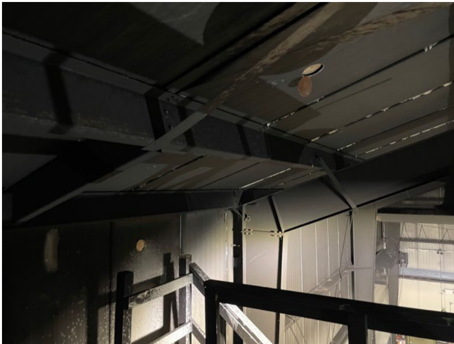
Heavy soot throughout warehouse.
