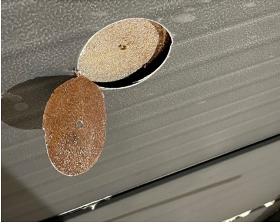
Ceiling panel delamination throughout building. Note dripping joint sealant.
