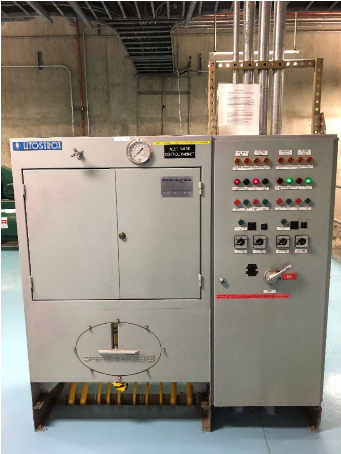
Inlet Valve HPU Control Cabinet
