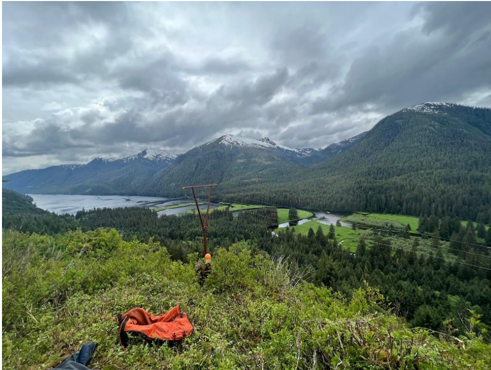
Contract Right-of-Way Clearing at STI Transmission Line at head of Carrol Inlet
