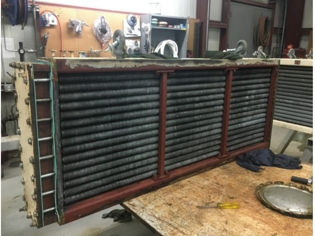
Freshly cleaned and serviced Swan Lake Generator Air Cooler
