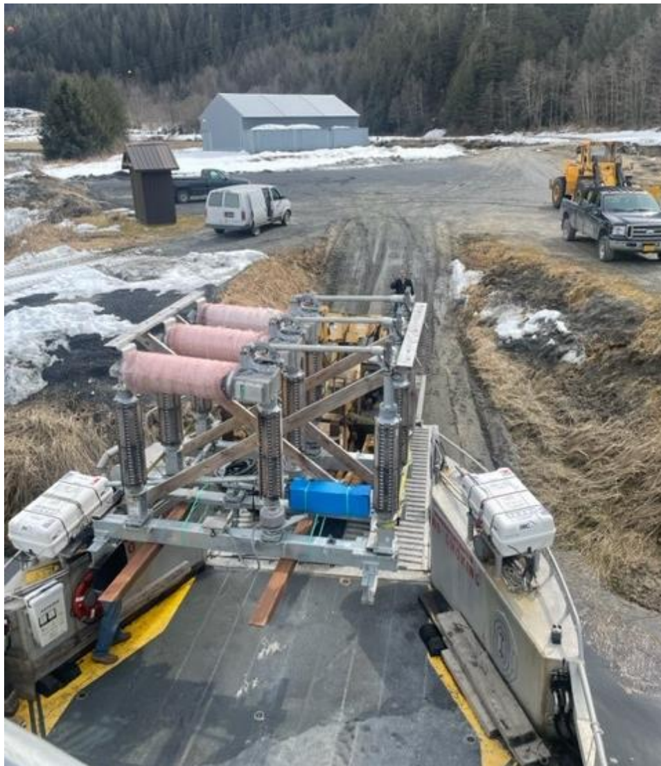
Circuit Switch Delivery to Tyee Plant
