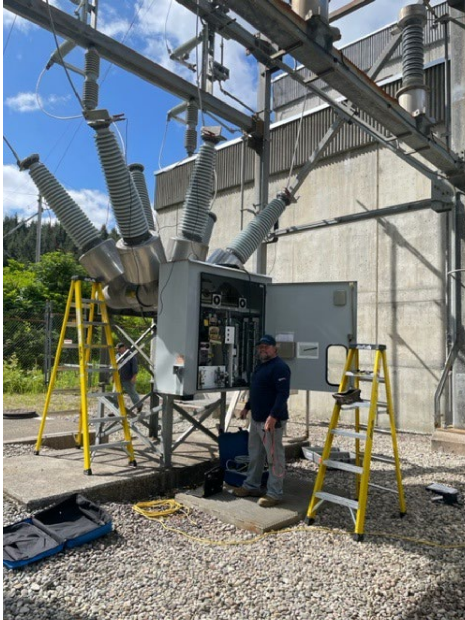
GCB-L1 Circuit Breaker Testing Swan Lake
