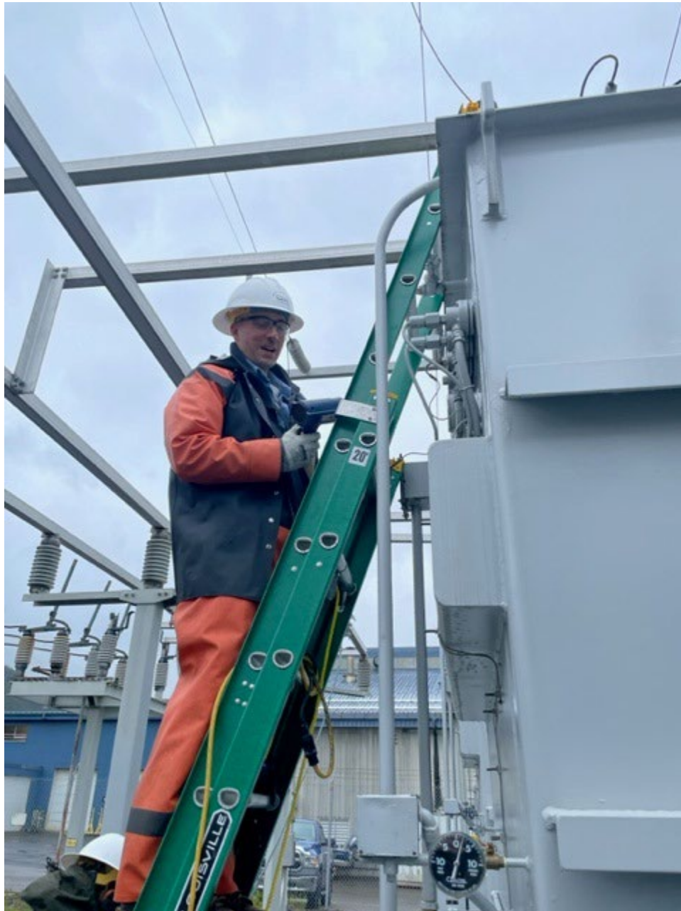
Swan Lake Electrician John Stanley Performing Work Orders (Bailey Substation)
