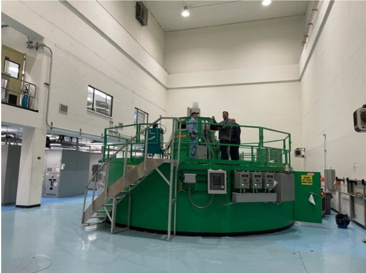
Kelly Consulting crew getting set up for DC Ramp Testing on Swan Unit S-1
