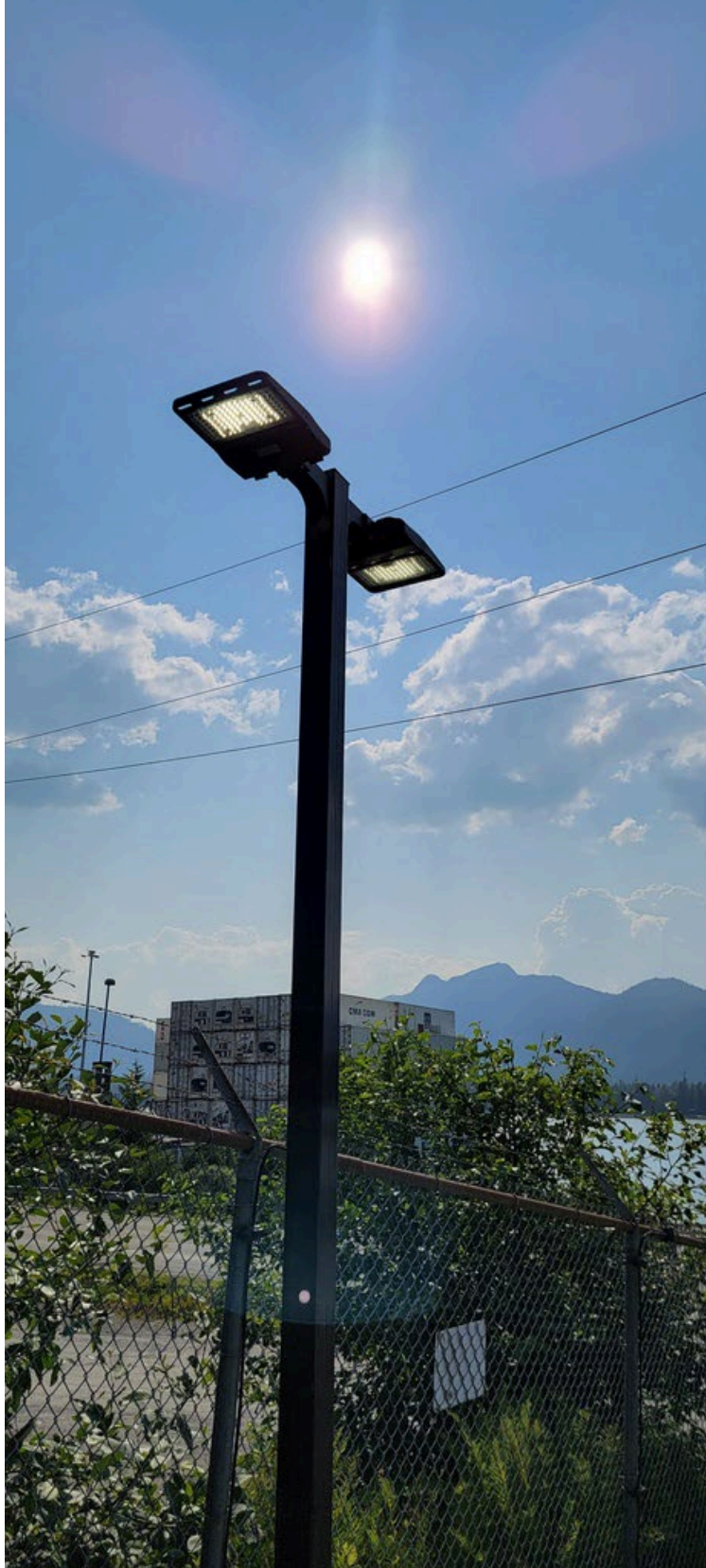
New Yard Lighting Petersburg Substation
