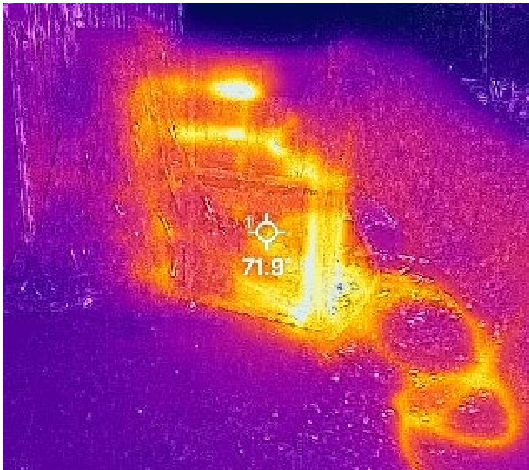
Thermal imaging view of filter station in service.
