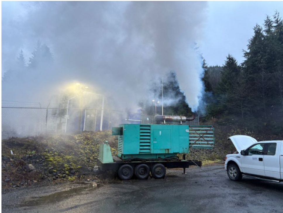
Petersburg's Rock-N-Road generator warming up to provide 480 volt power.
