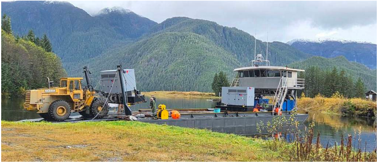
New E-Gen delivery to Tye Lake. Part of the new Station Service Project, these are the two new Generators that will be mounted outside the Tye Plant to provide automatic emergency standby power in the event of a full plant outage.
