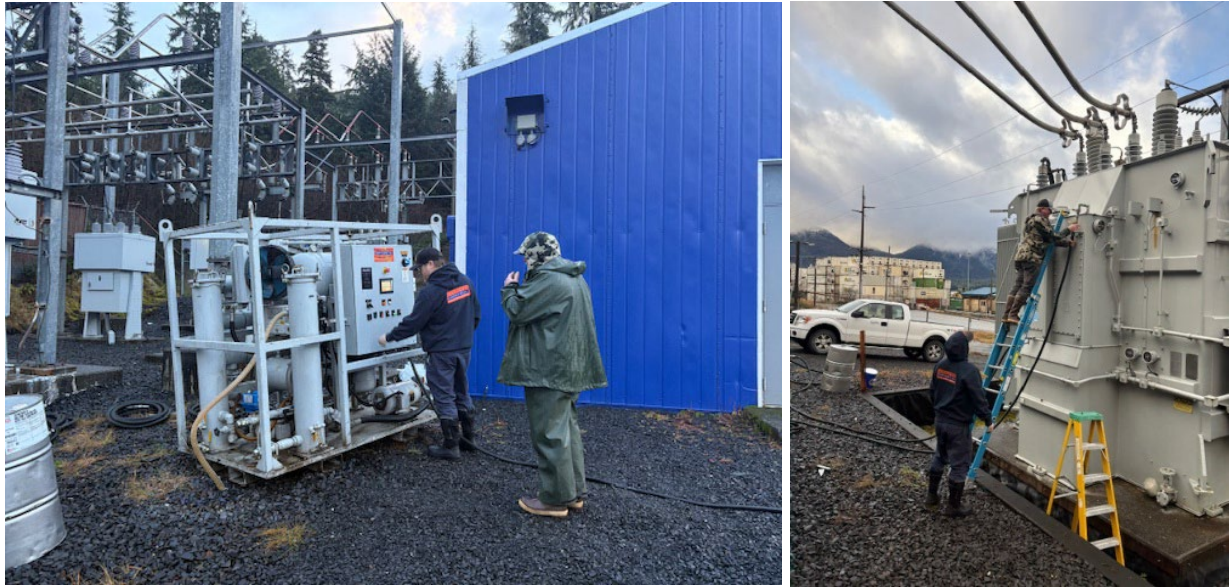
Tyee Electrician, Ashley Goynes, and Equipment Rep, Justine Lane, hooking up the Unit.
