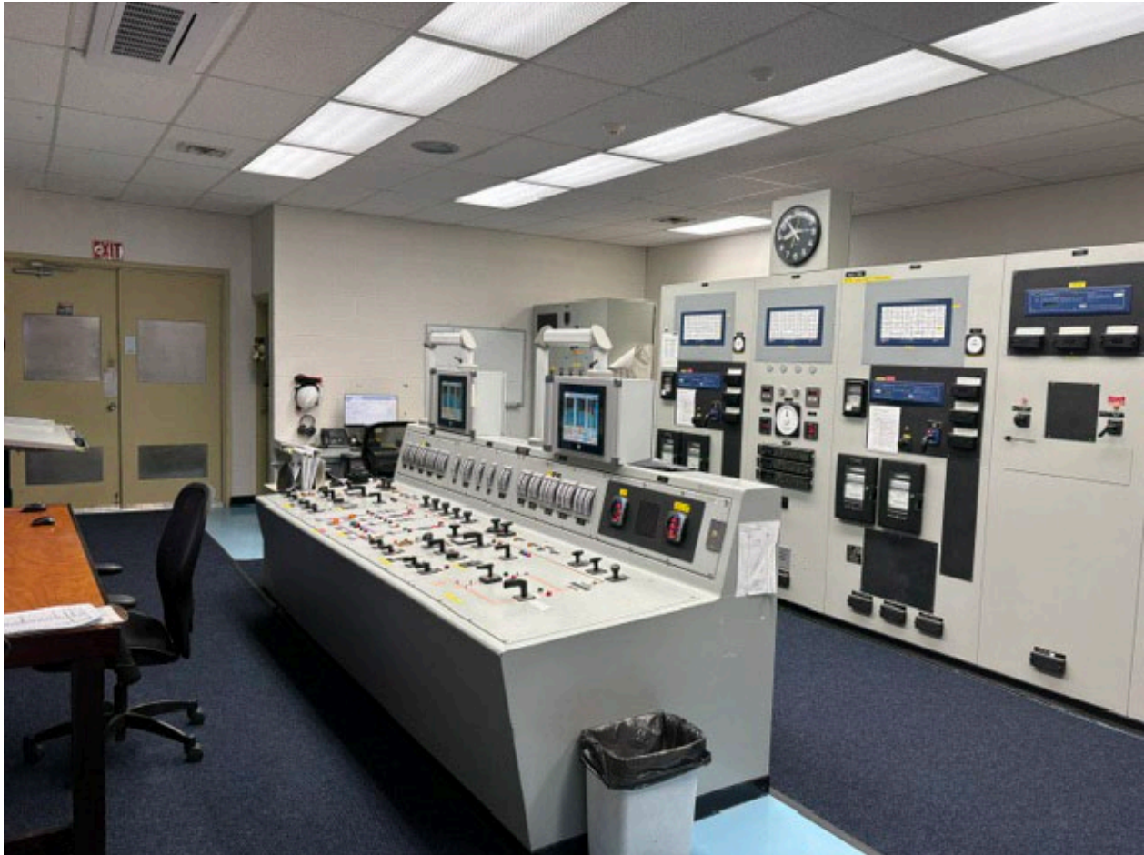
Above: Swan Lake Bench Board Inside Newly Sound Proofed Control Room
