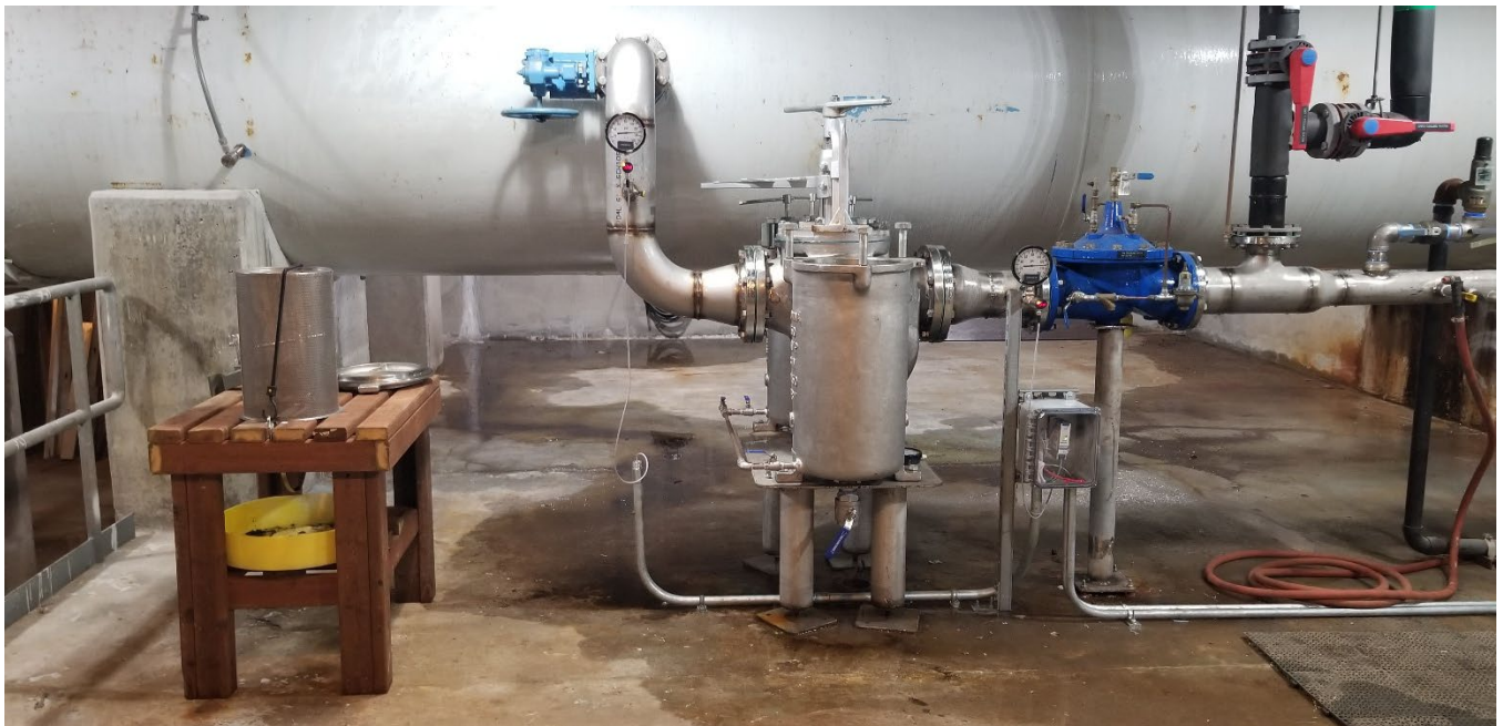
Swan Cooling Water Strainer with cleaning station and New Remote Pressure Monitoring Equipment.
