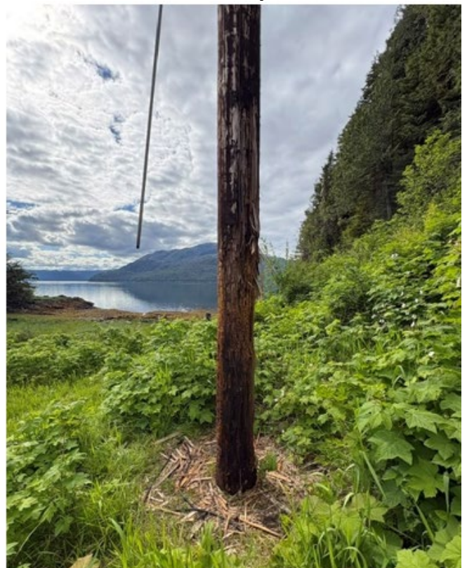
Below: Close-up of Bear-scratched Antenna Pole behind Battery Stand
