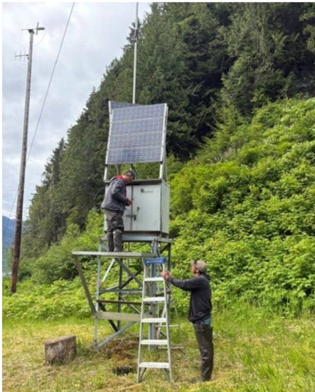
Below: Comms testing at Marine Radio Solar Panel
