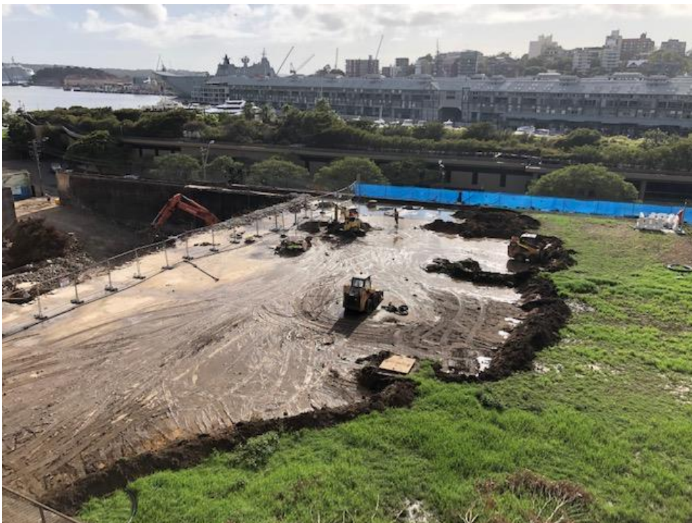
Photo 2: Removal of asbestos contaminated soil on top of the former fuel bunkers
