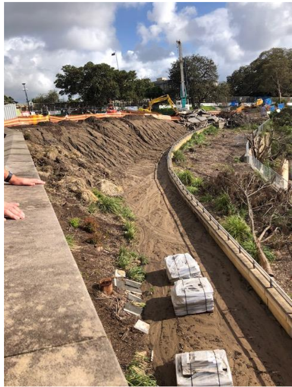
Photo 4: Stockpiles in the center of the site – lack of erosion and sediment controls evident
