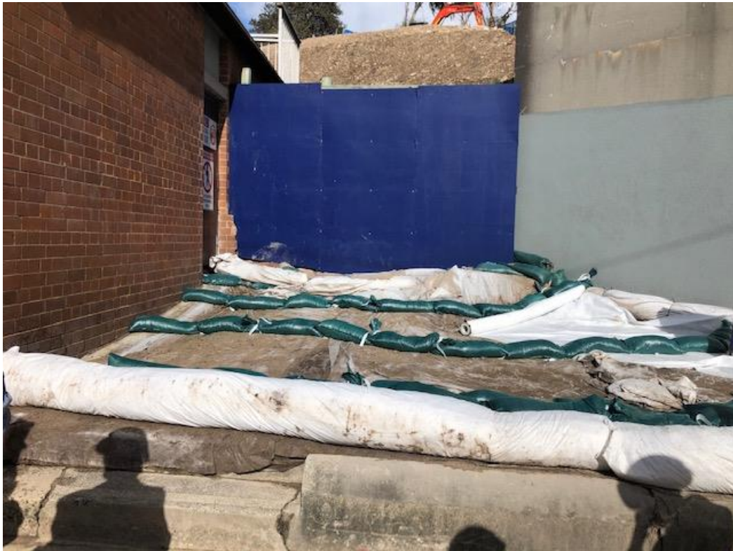
Photo 12: Erosion and sediment controls adjacent Lincoln Crescent site access
