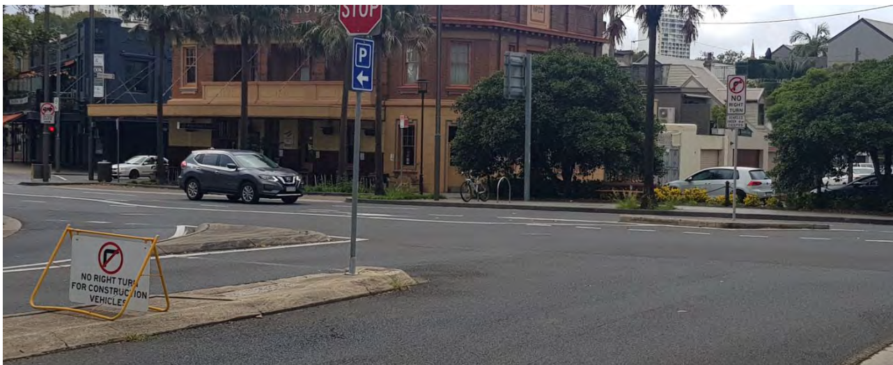
Photo 10: Signage for construction vehicles, following several nonconformities
