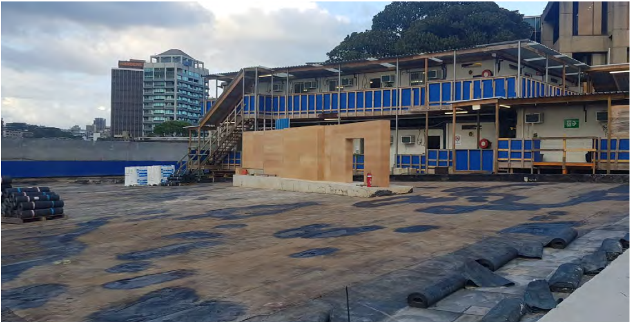
Photo 2: Sealing the surface over the Eastern Distributor with sandstone block work being erected.
