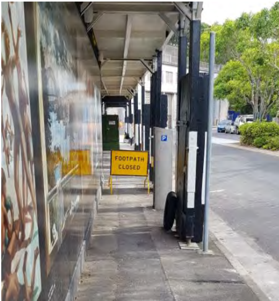
Photo 8: Closed footpath without adequate detour.
