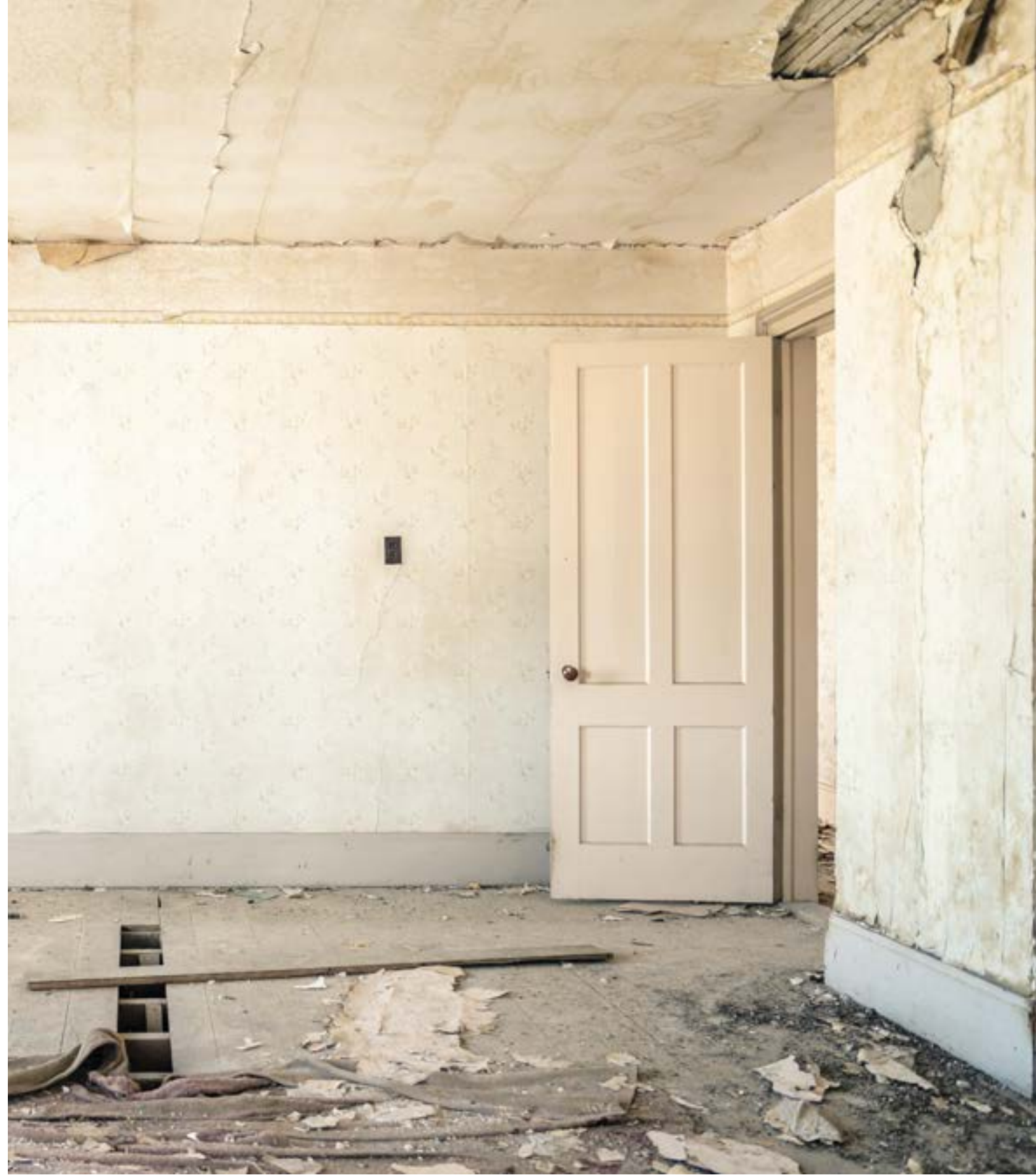
Salvaged Building Materials: Urban mining allows for the recovery and reuse of materials from demolished or renovated buildings. This includes items like doors, windows, flooring, bricks, and timber, which can be repurposed in new construction projects.
