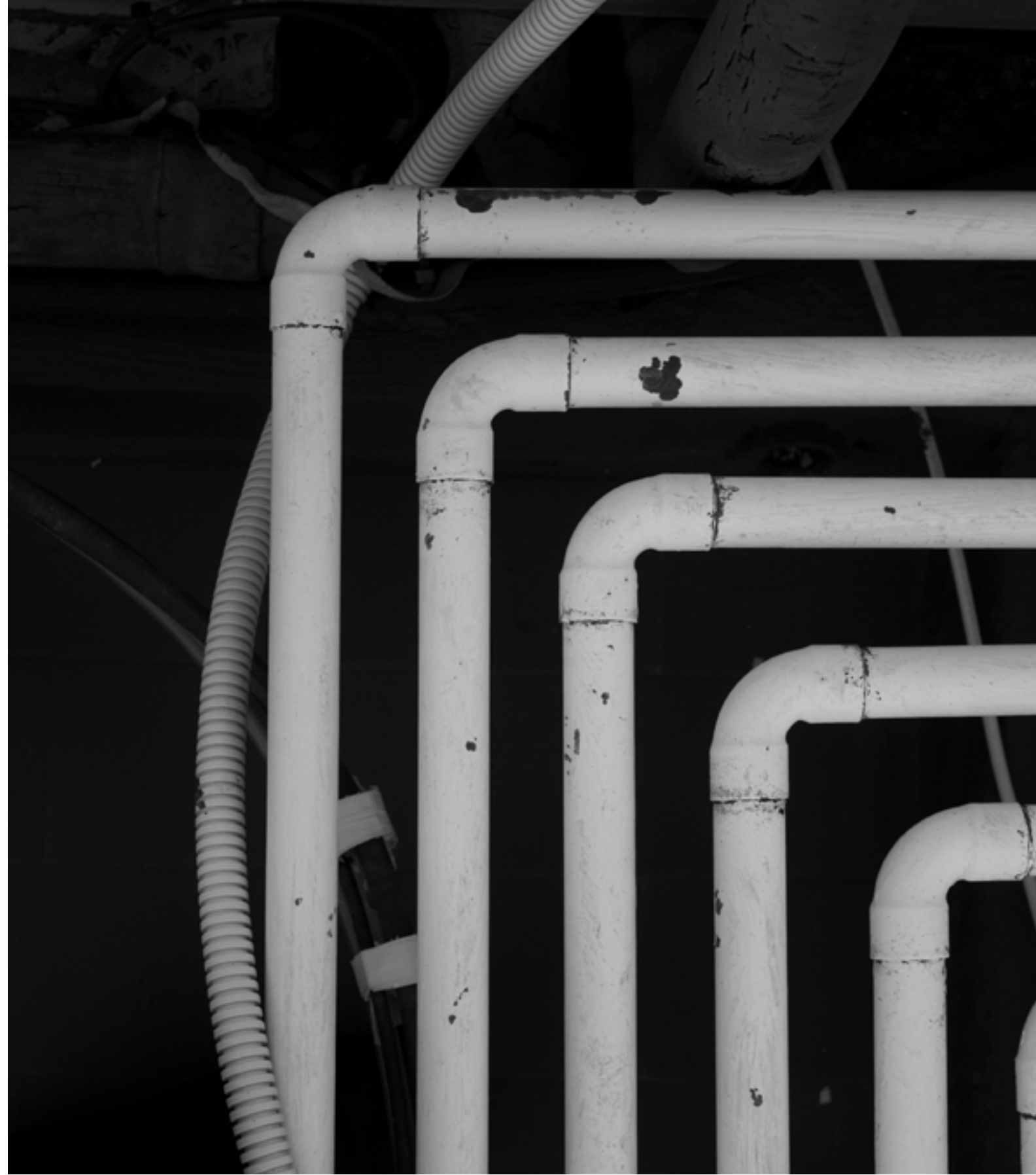
Building Systems: Urban mining enables the retrieval and refurbishment of building systems, including mechanical, electrical, and plumbing components. These systems can be tested, repaired, and reintegrated into new architectural projects, reducing waste and promoting efficient resource utilization.
