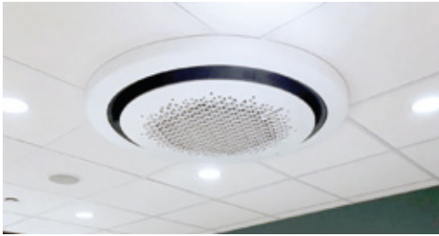
Plasma Air model PA664 was installed in multiple VRF round cassettes and ducted air handling units.
