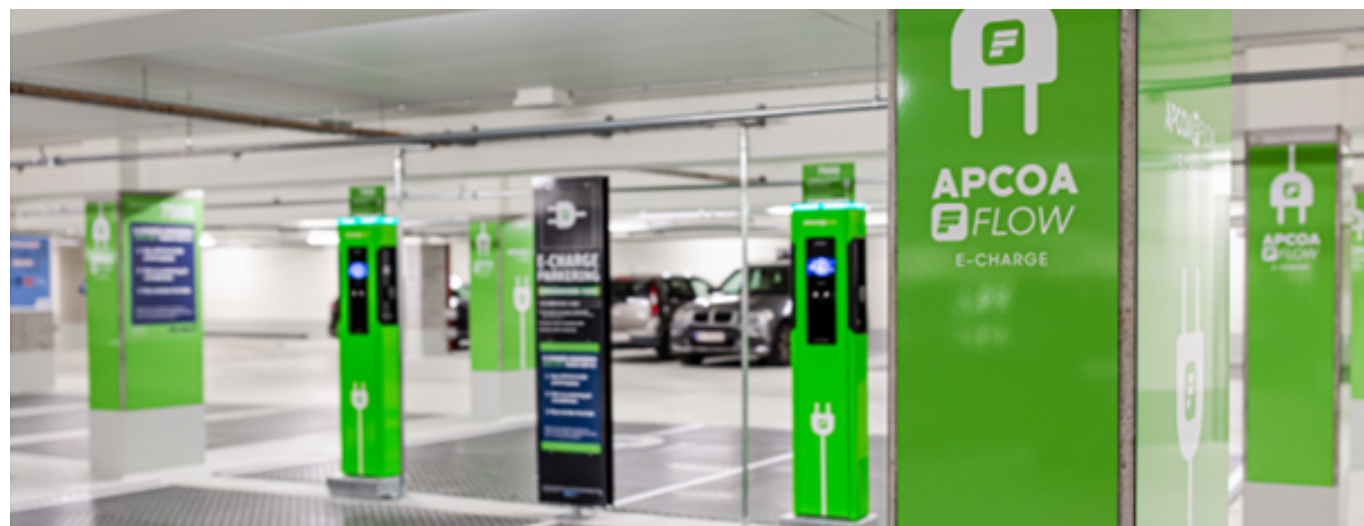
Abb. 18: APCOA Parking Denmark (2022), EV Charging
