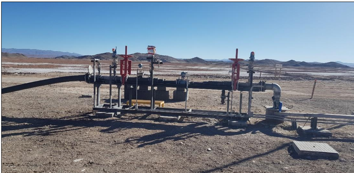
Figure 16-9 – Production Well SVWP21-02.
