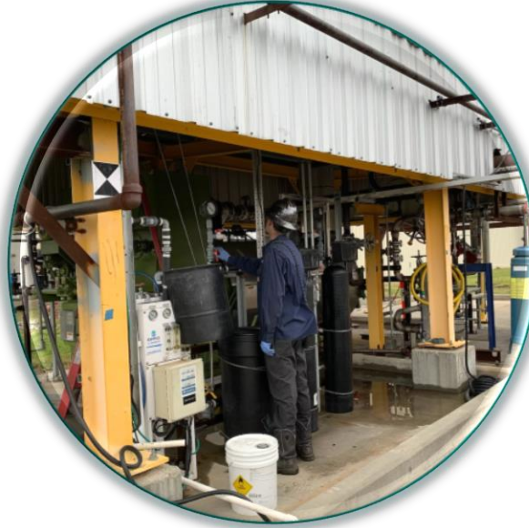
Water Treatment Plant at Vidalia
