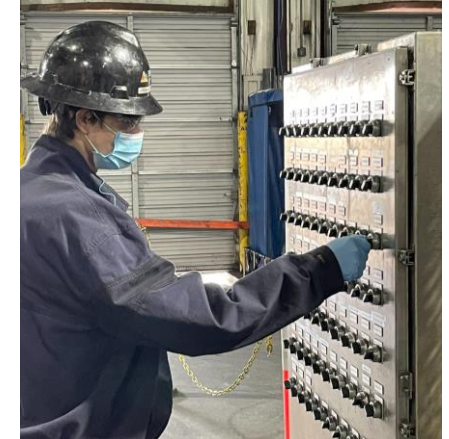
Vidalia employee operating the gravity drain tank
