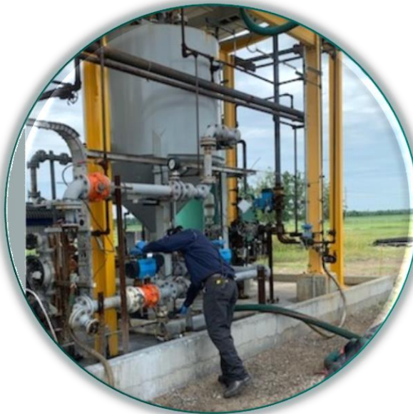
Water neutralisation skid in Vidalia
