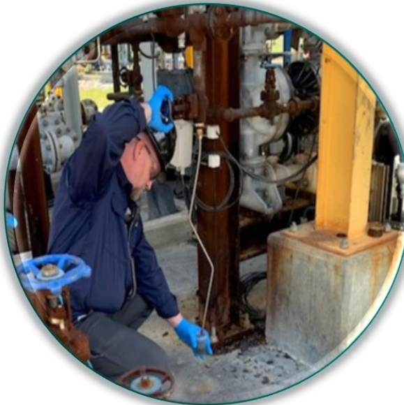
Water sample being taken for testing in Vidalia
