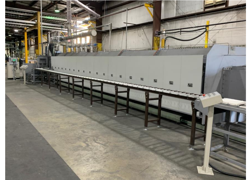
Carbonisation furnace main chamber
