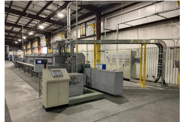
New pilot carbonisation furnace control station
