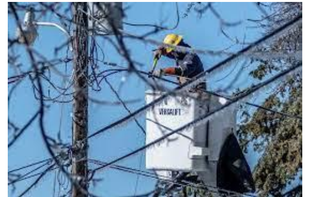
Power outages resulting from severe winter storms
