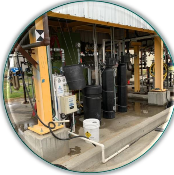
Water Treatment Plant at Vidalia
