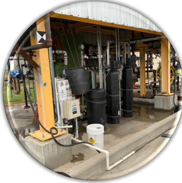
Water Treatment Plant at Vidalia
