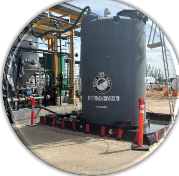
Water treatment plant at Vidalia
