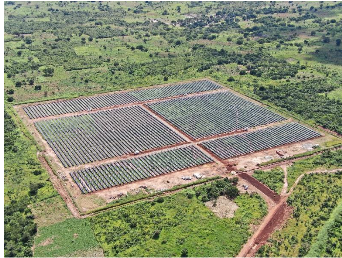
Figure 1: Balama Solar Battery System development.
