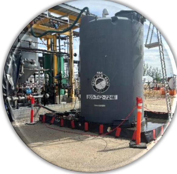
Water treatment plant at Vidalia
