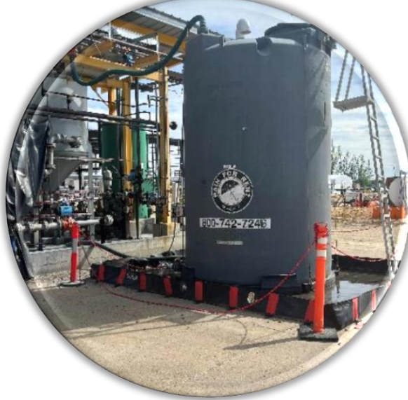
Water treatment plant at Vidalia
