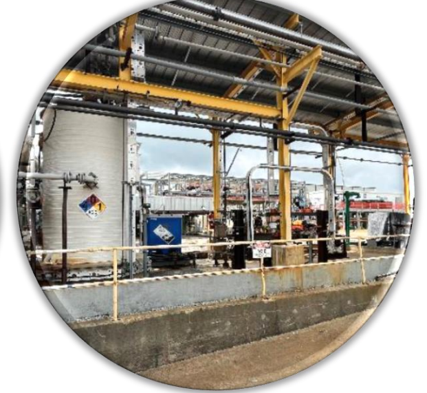
Phase 1 acid neutralisation plant at Vidalia
