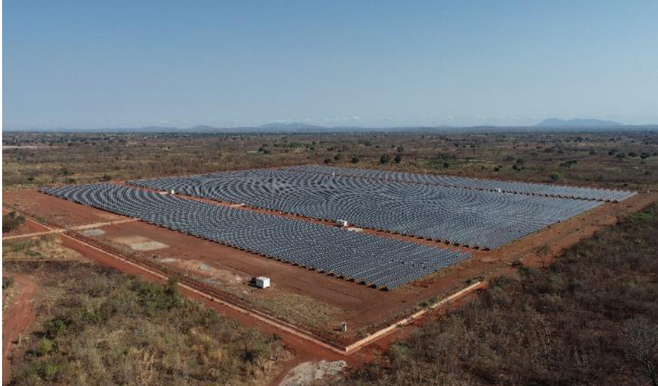
11.25 MWp solar photovoltaic array
