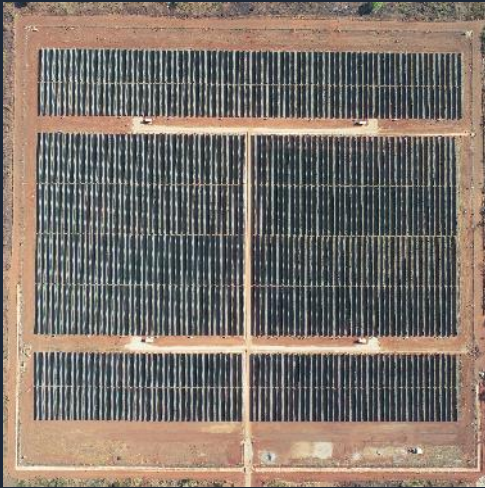
Balama solar photovoltaic system
