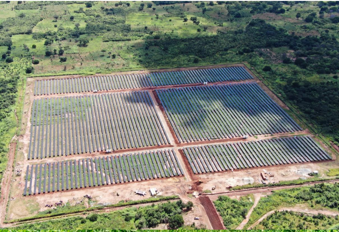
► Balama solar photovoltaic system
