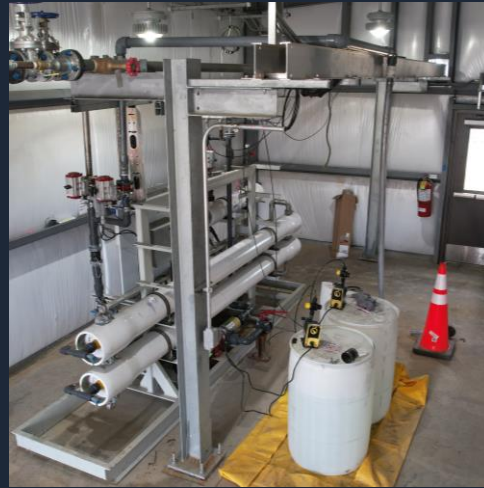
Reverse osmosis plant at Vidalia
