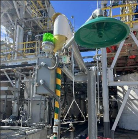
Greenlight illumination on safety shower wiring at Vidalia
