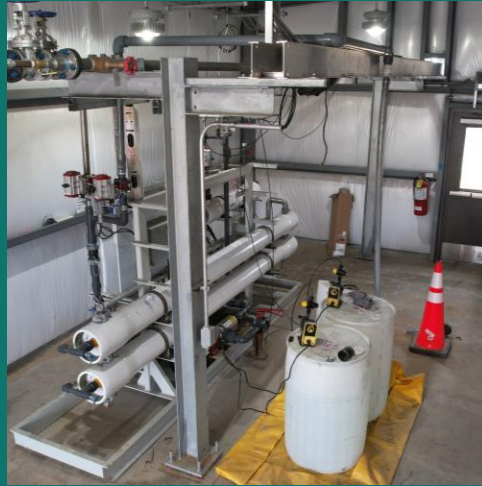
Reverse osmosis plant at Vidalia
