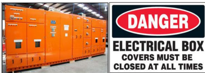
Coloured Electrical Cabinets
