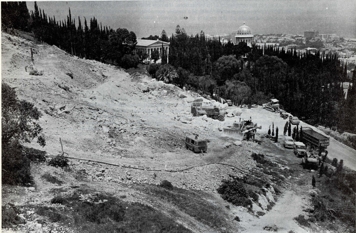
Beginning of the excavation of the site, on the arc, of the permanent seat of the Universal House of Justice. July 1975.
