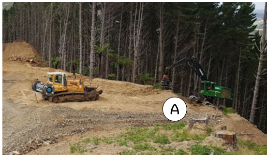
A Ropes are carving through bund and landing fill
