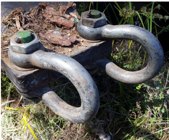
Cable attachment points engineered for the expected loads.
